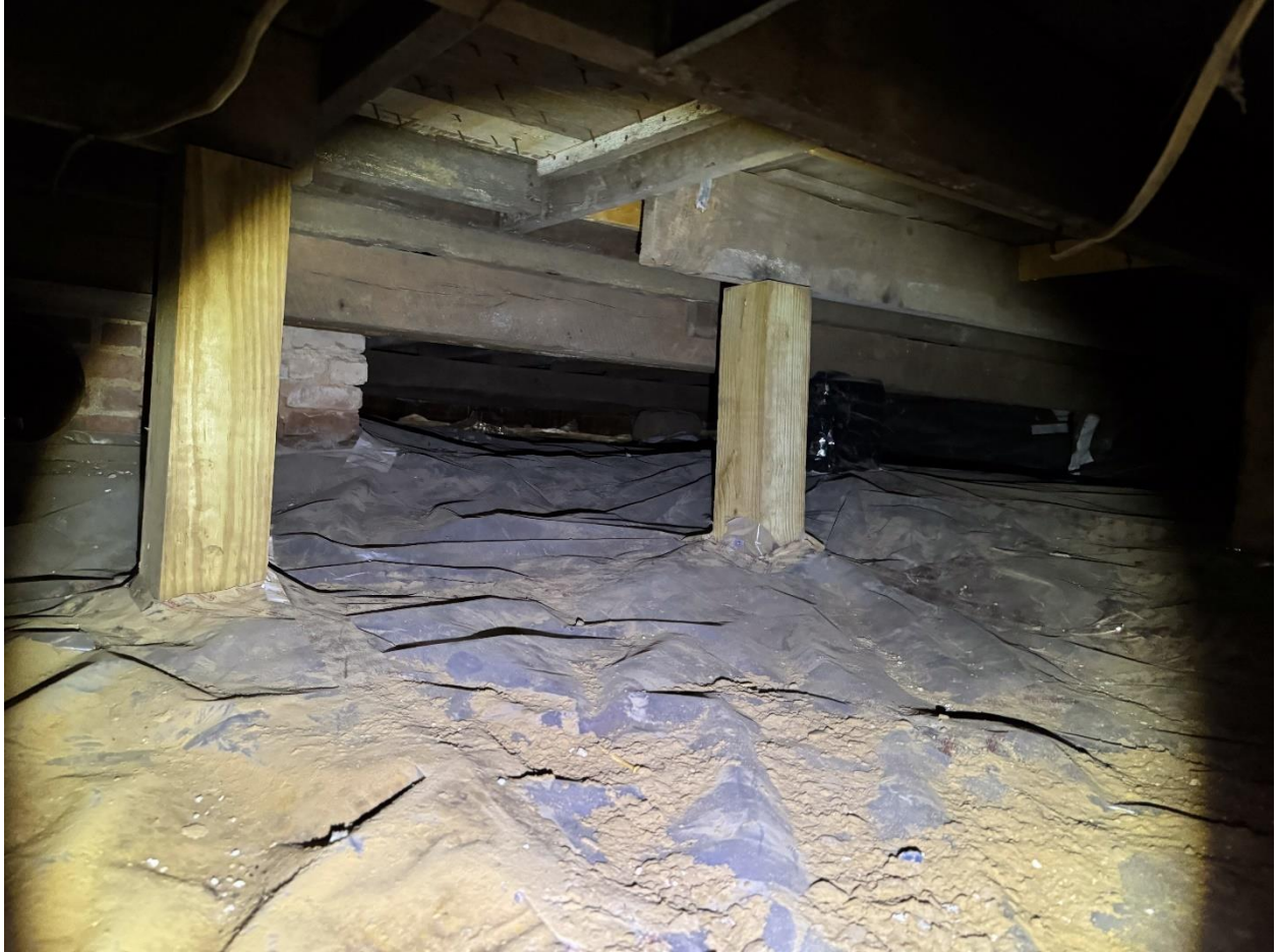
Figure 14 View at the crawlspace looking northeast. Visible are the original wood timber beams.
