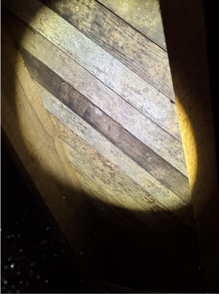
Figure 15 Looking up at the wood plank subfloor and wood joists at the west portion of the Caldwell-Bradford School in the crawlspace. This section was likely added later when the former school was converted into a residence.
