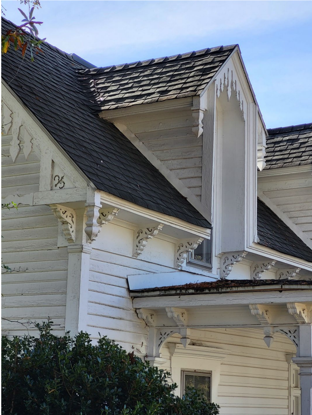
Detail of front elevation gabled dormer with illustrative ornamental sawnwork, pendills, and brackets that appear on all four elevations.
