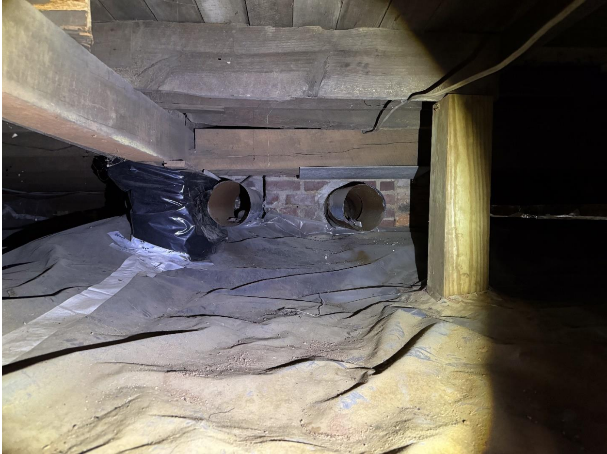
Figure 13 View at the crawlspace looking north toward the brick chimney. The wood plank subfloor at the top of the photo runs perpendicular to the floor beams, identifying this portion of the Caldwell-Bradford School as the original portion.
