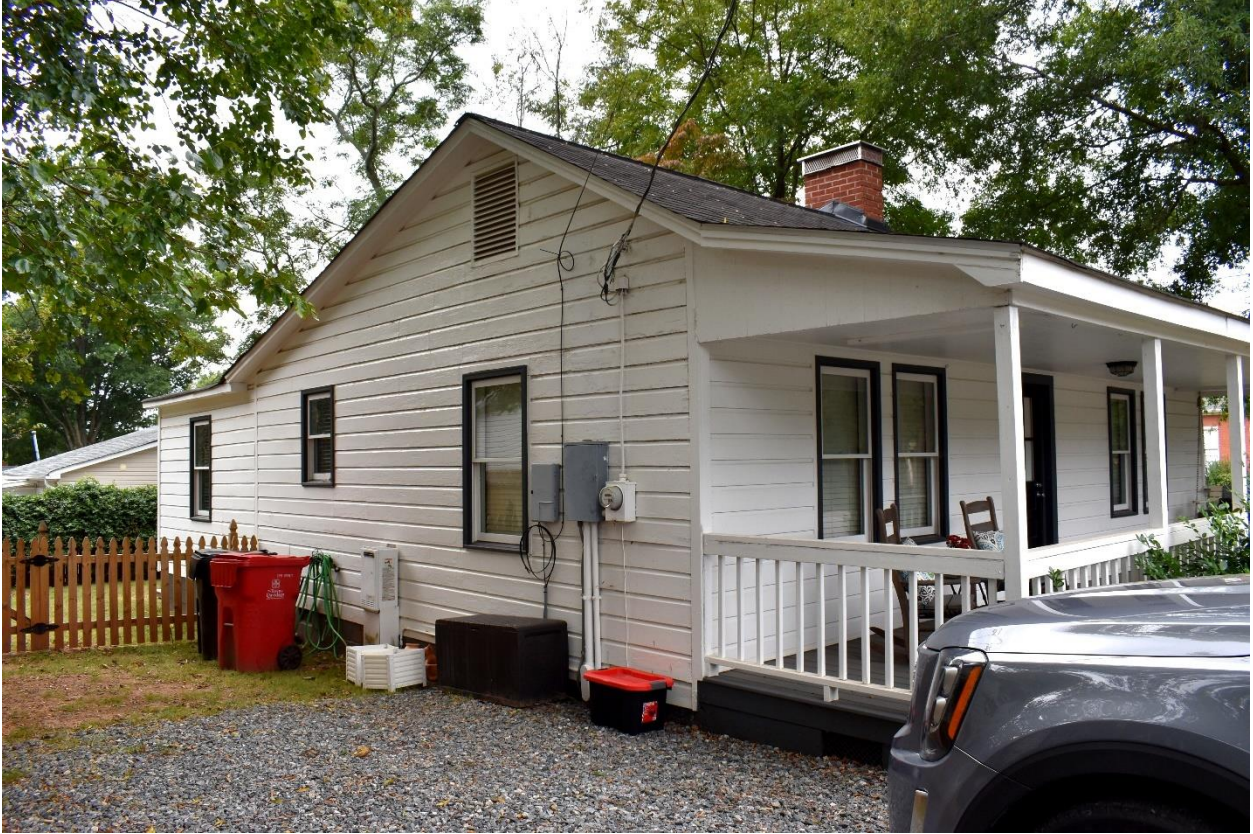
The east elevation of the Armour Street Mill House is similar to the west elevation at the first and second bays. However, the third bay has a shorter 1/1 vinyl window. The gabled addition at the rear is flush with this elevation and has a typical window centered in its face. Alongside this elevation is a narrow gravel parking area and wood picket fence.
