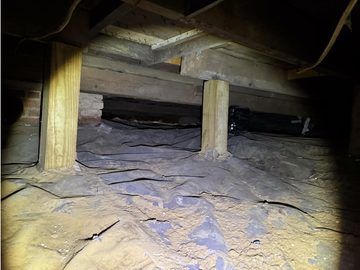
Figure 13 View at the crawlspace looking northeast. Visible are the original wood timber beams.
