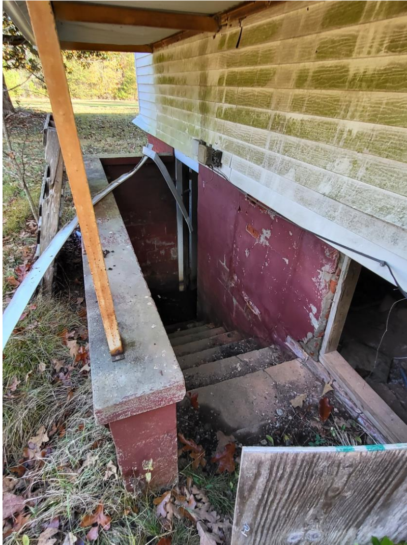
Detail of covered rear elevation stairwell leading to crawl space and basement.
