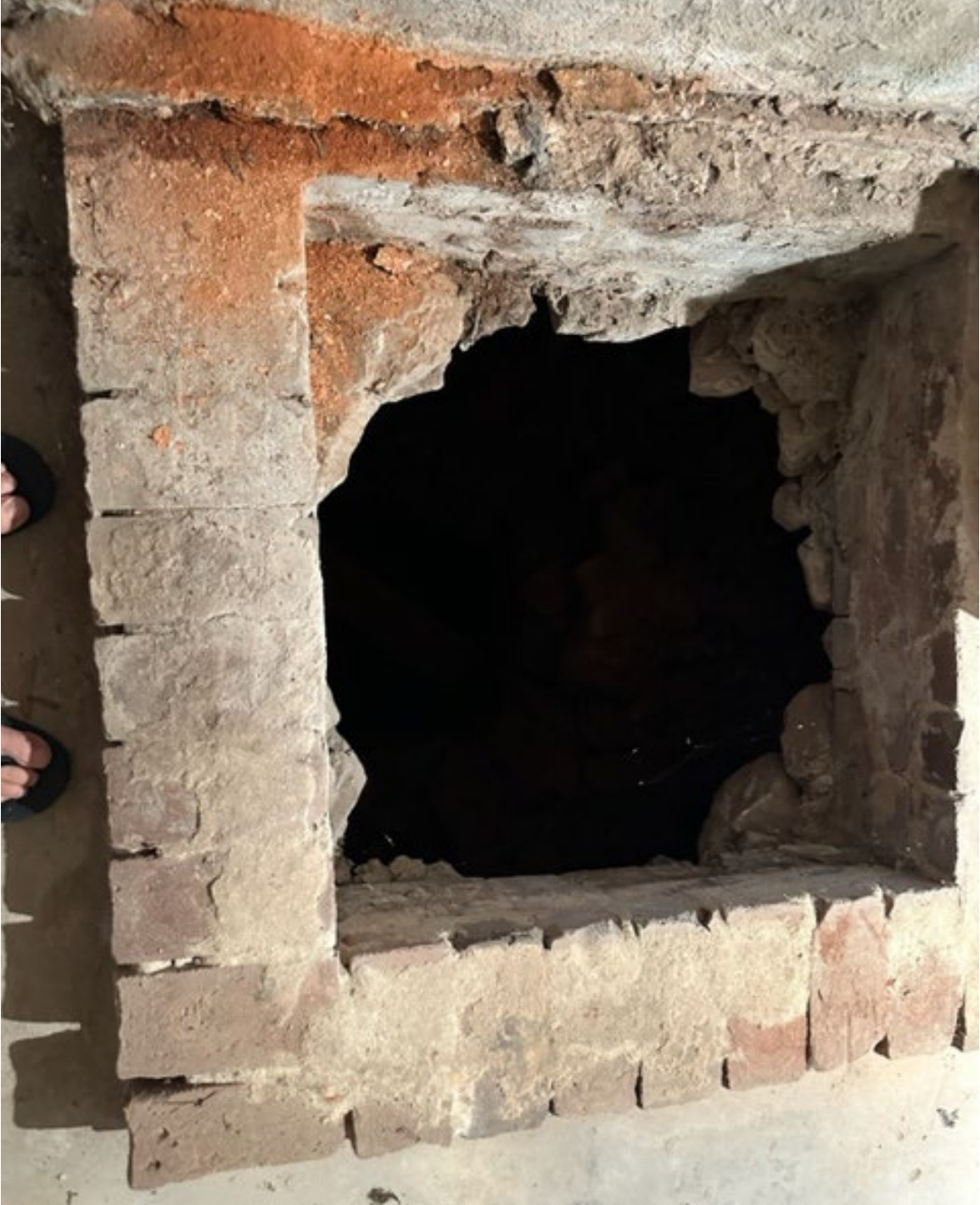
Above: Close-up view of exterior of original brick well in Southeast basement room.
