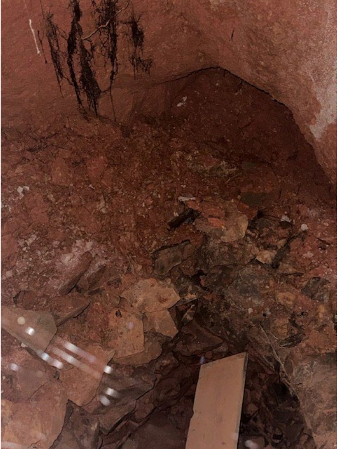
Above: View of cavern within original brick well in Southeast basement room.
