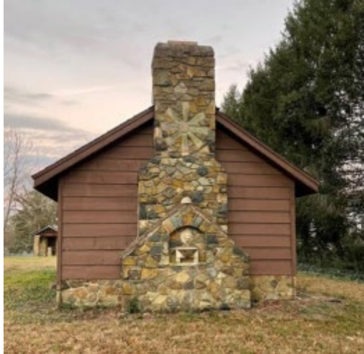
Rear elevation of Summer House at Akers Acres. Source: Dr. Timothy Brown.
