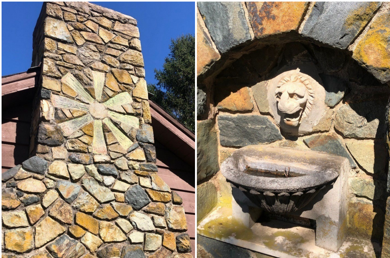
Exterior chimney details of Summer House at Akers Acres. Source: Roger Ball.
