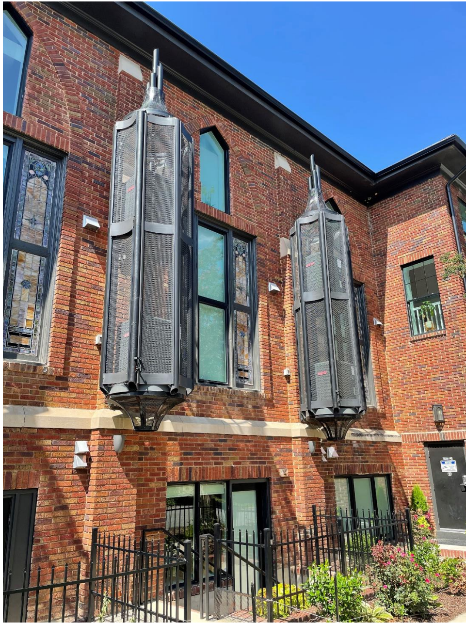
Figure 16 Typical heat pump surround at east elevation, 2023.
