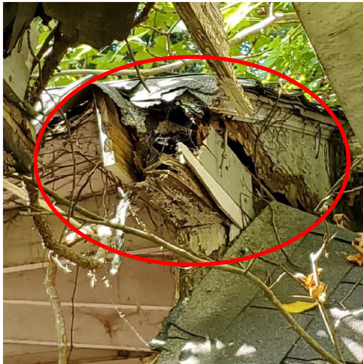
Photograph 32: View of water and/or insect related damage to porch framing (oval).
