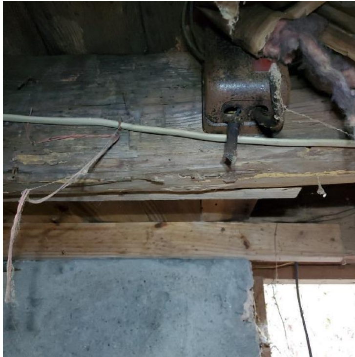
Photograph 71: View of potential insect related damage.
