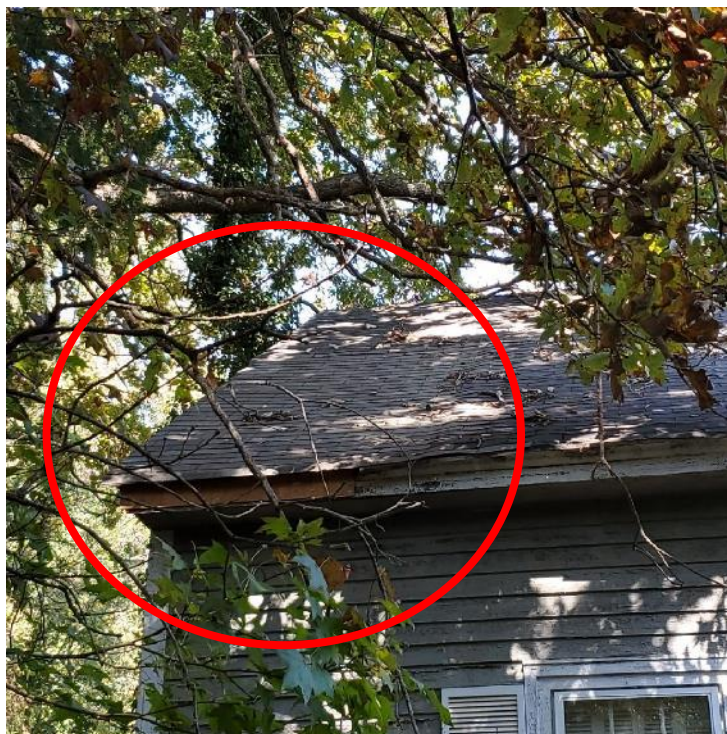
Photograph 22: View of different color shingles and replaced fascia at southwest corner (oval).
