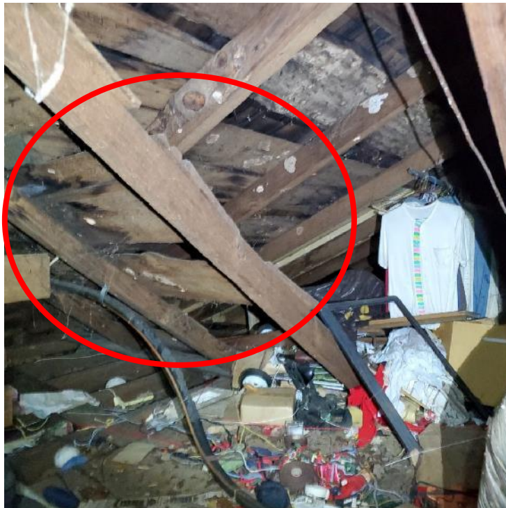
Photograph 38: View of water-related staining at original to rear portion roof transition (oval).
