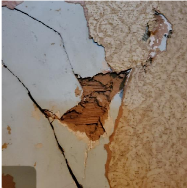
Photograph 41: View of wall construction at failed interior finish location.
