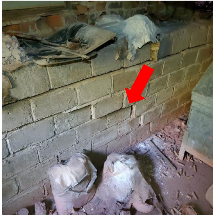
Photograph 53: View of cracking and out of plane displacement of crawlspace CMU retaining wall (arrow).
