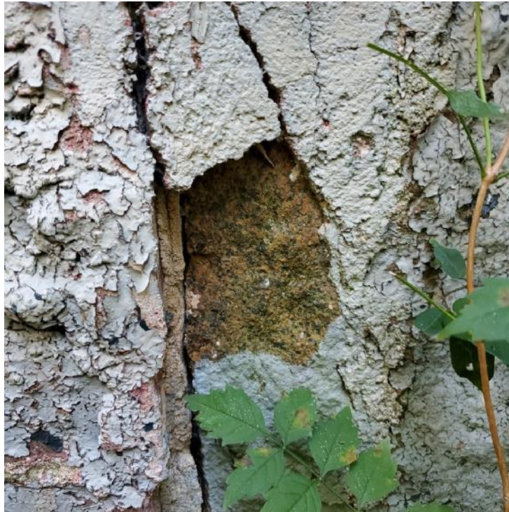
Photograph 21: Close-up view of delamination on the exterior face of the mass stone pier along the south elevation.
