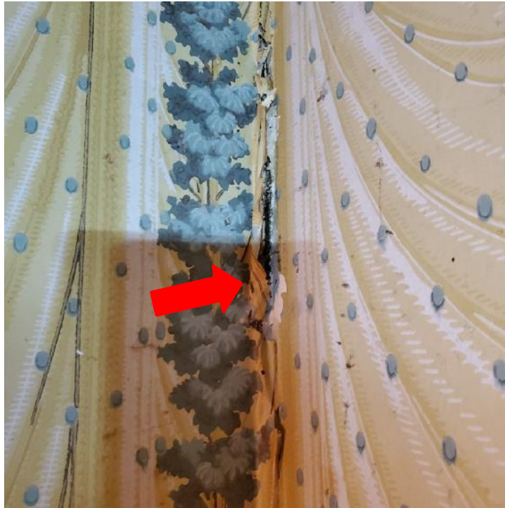
Photograph 47: View of torn wallpaper at southeast corner of bathroom addition (arrow).
