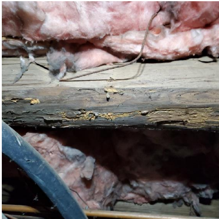
Photograph 72: View of potential insect related damage (oval).
