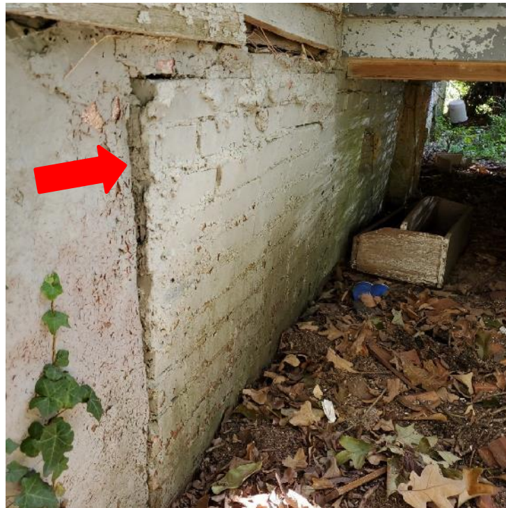
Photograph 18: View of vertical displacement of brick infill adjacent to the front porch (arrow). Note the paint along the side of the exposed brick.
