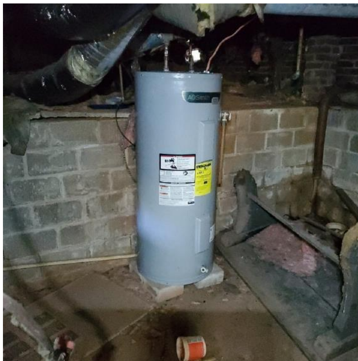
Photograph 52: View of lowered crawlspace floor in the rear portion of the crawlspace.
