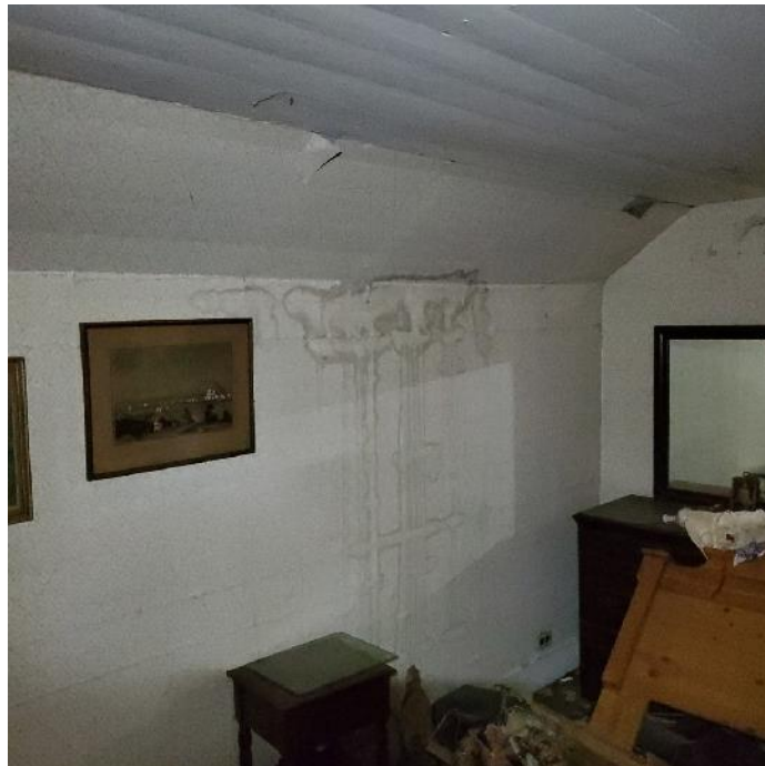
Photograph 36: View of water-related staining on wallpaper.
