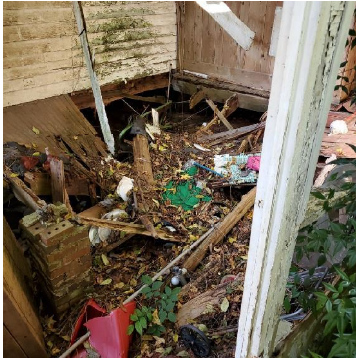
Photograph 29: View of collapsed porch floor.
