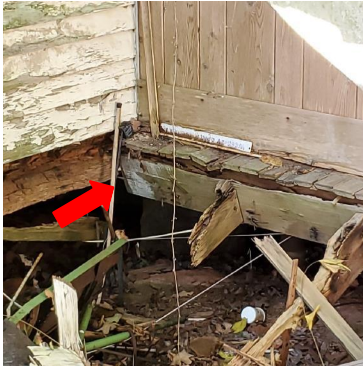
Photograph 31: View of failed joist connection below bathroom addition (arrow).
