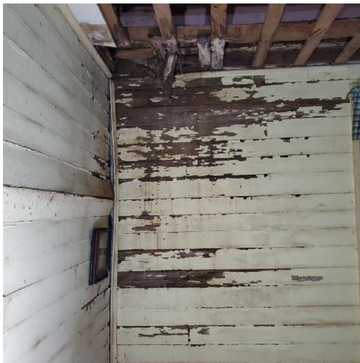
Photograph 50: View of water-related staining and damage in bedroom at north end of the rear portion of residence.
