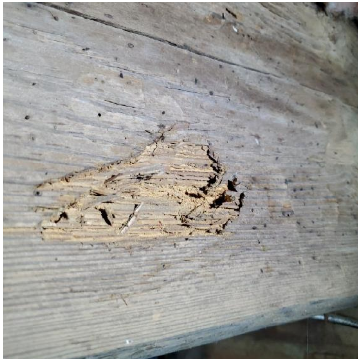
Photograph 74: Close up view of potential insect related damage.
