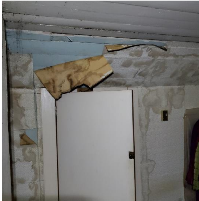
Photograph 35: View of water-related staining on wallpaper.
