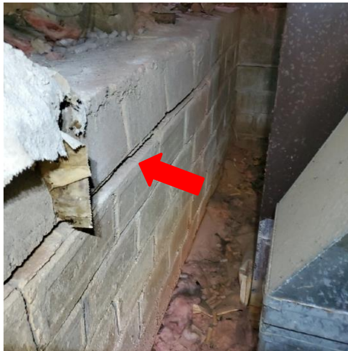
Photograph 54: View of cracking and out of plane displacement of crawlspace CMU retaining wall (arrow).
