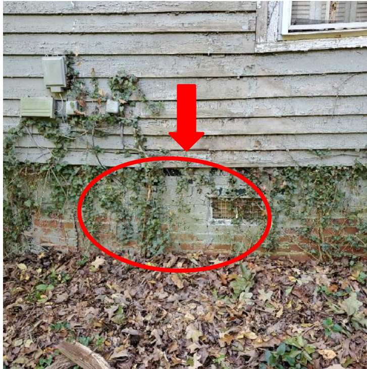
Photograph 25: View of sag in siding at the first-floor level along the west elevation of the rear portion of the residence (arrow). Note the step crack in the brick masonry infill (oval).
