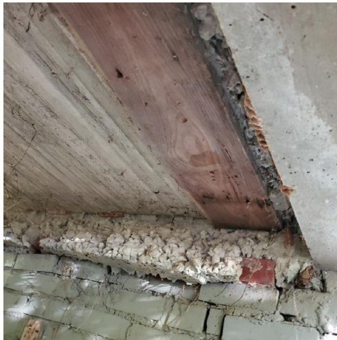
Photograph 16: View of front porch CIP concrete slab bearing on brick masonry infill.
