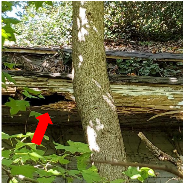
Photograph 34: View of water and/or insect related damage to porch framing (arrow).
