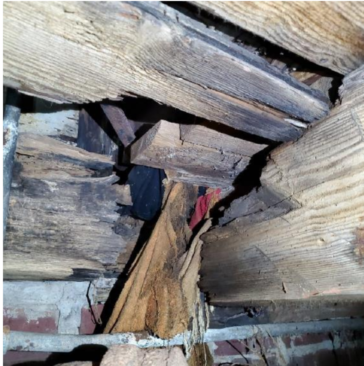
Photograph 67: View of insect and/or water related damage, see additional photo above.
