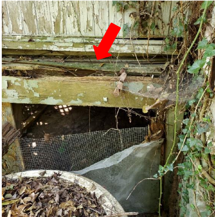
Photograph 33: View of water and/or insect related damage to porch framing (arrow).
