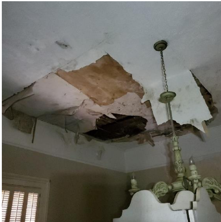
Photograph 42: View of water related damage to the ceiling at the southwest corner.
