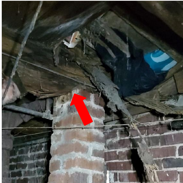
Photograph 63: View of brick pier at location of insect and water related damage to flooring. Note the crushed beam at the pier bearing (arrow).
