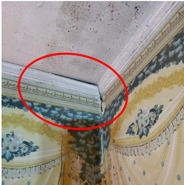
Photograph 46: View of gap between ceiling finishes and wall trim (oval).
