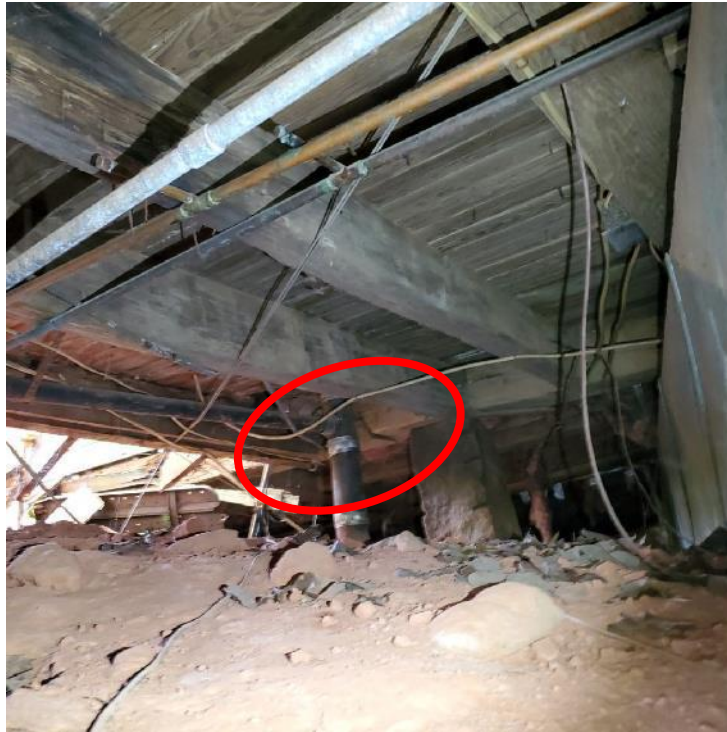
Photograph 61: View of porch framing below bathroom addition. Note the distress of the floor framing at the beam to girder connection (oval).
