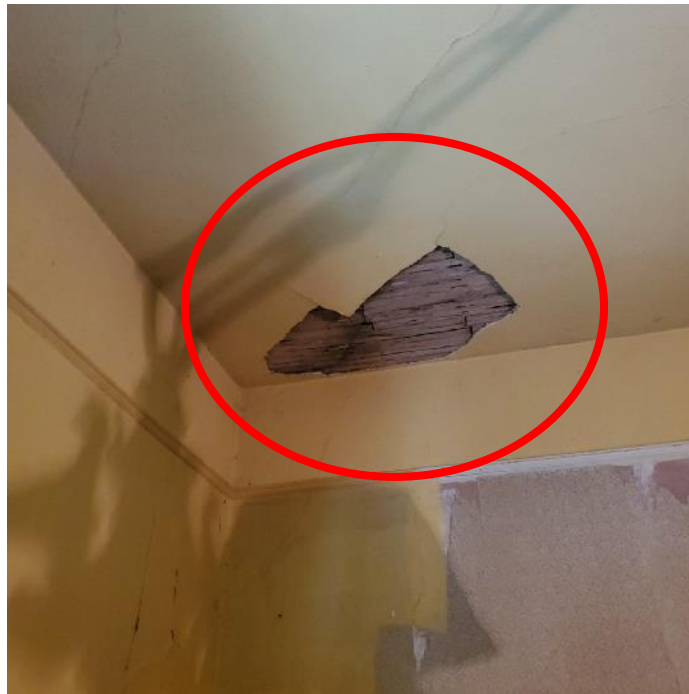
Photograph 43: View of failed ceiling finishes at the southeast corner (oval).
