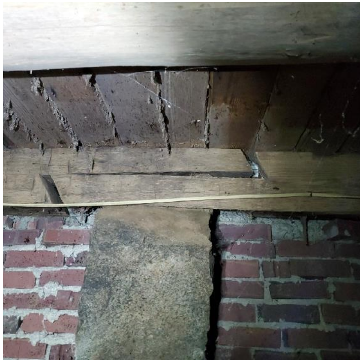
Photograph 60: View of potential movement at girder lap splice.
