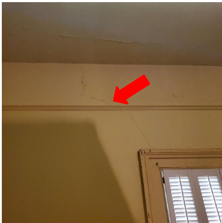
Photograph 40: Representative view of cracking within interior finishes of the original portion of the residence (arrow).
