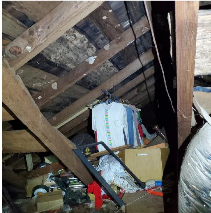
Photograph 37: View of storage in attic space at original to rear portion transition.
