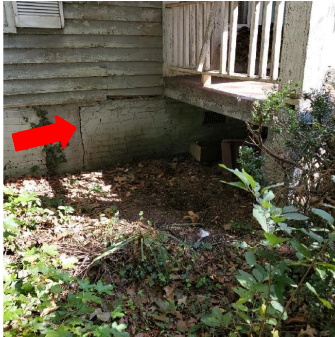
Photograph 17: View of vertical displacement of brick infill adjacent to the front porch (arrow).
