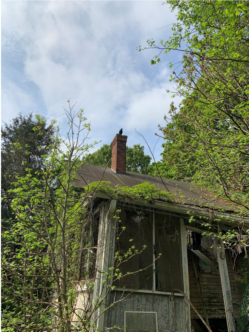
Collapsed rear porch
