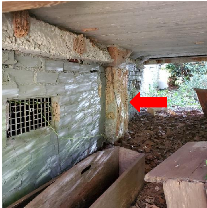
Photograph 19: View of mass stone pier located along south elevation porch slab bearing (arrow).
