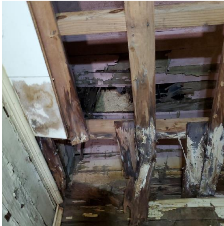
Photograph 51: View of water-related staining and damage in bedroom at north end of the rear portion of residence.
