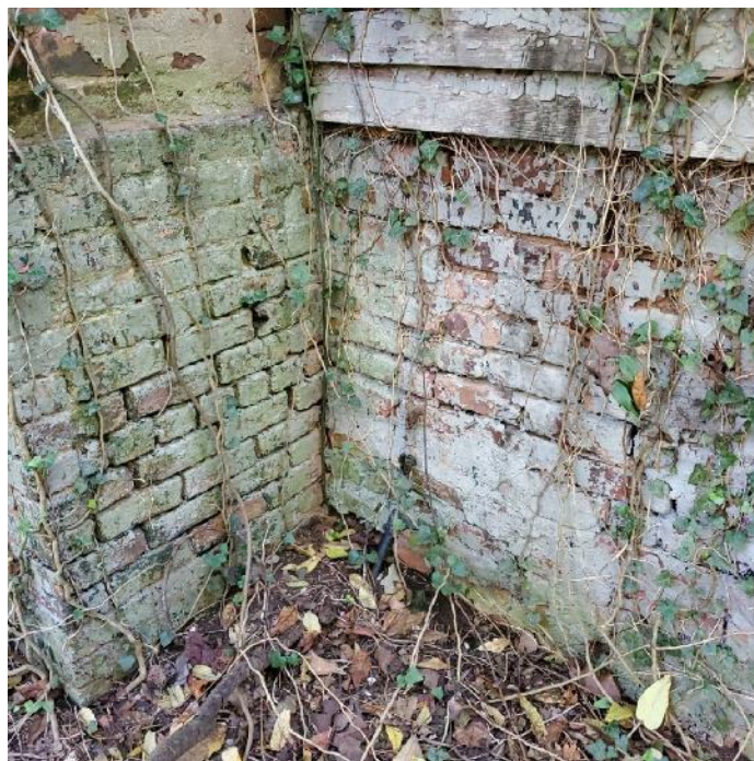
Photograph 26: View of recessed mortar joints in brick infill masonry and in the exterior chimney masonry.
