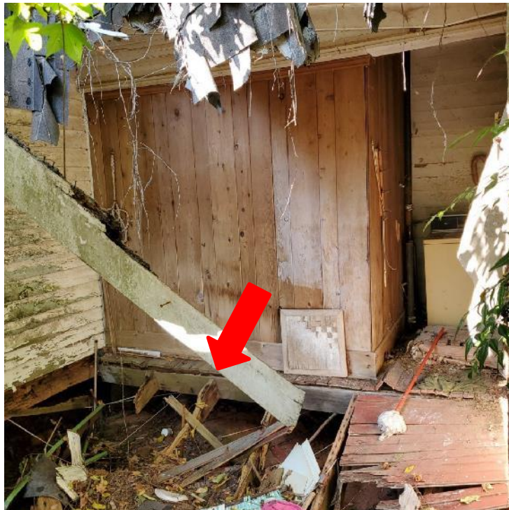
Photograph 30: View of bathroom addition located above the porch framing (arrow).
