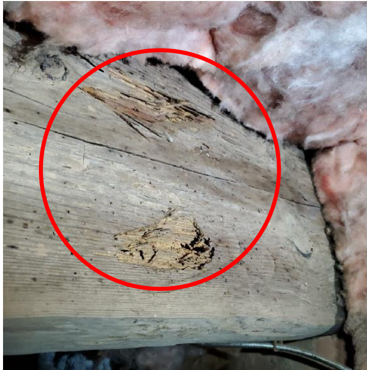
Photograph 73: View of potential insect related damage (oval).
