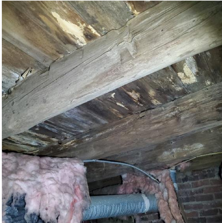
Photograph 75: View of moisture related damage at wood flooring.
