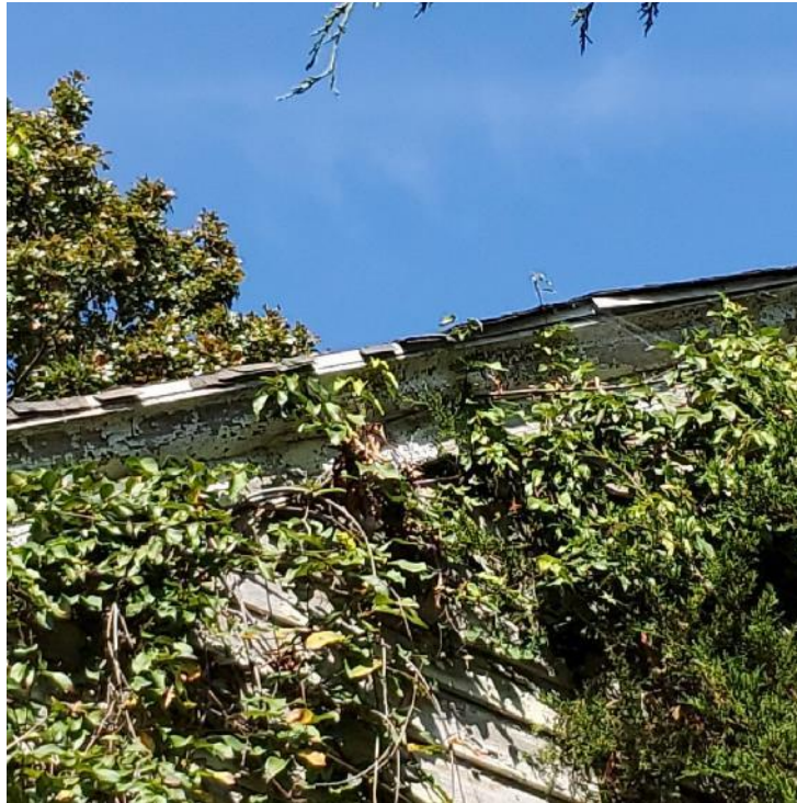
Photograph 13: View of vegetative growth along east elevation of original portion of residence.
