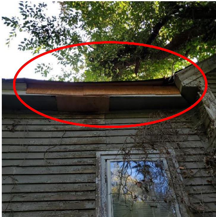
Photograph 24: View of plywood at fascia along the west elevation of the rear portion of the residence (oval).
