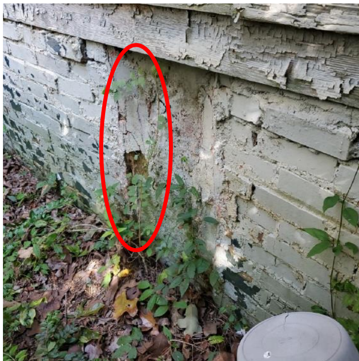
Photograph 20: View of delamination on the exterior face of the mass stone pier along the south elevation (oval).
