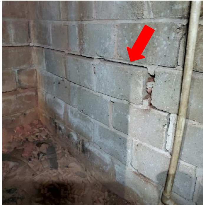
Photograph 55: View cracking and out of plane displacement of crawlspace CMU retaining wall (arrow).
