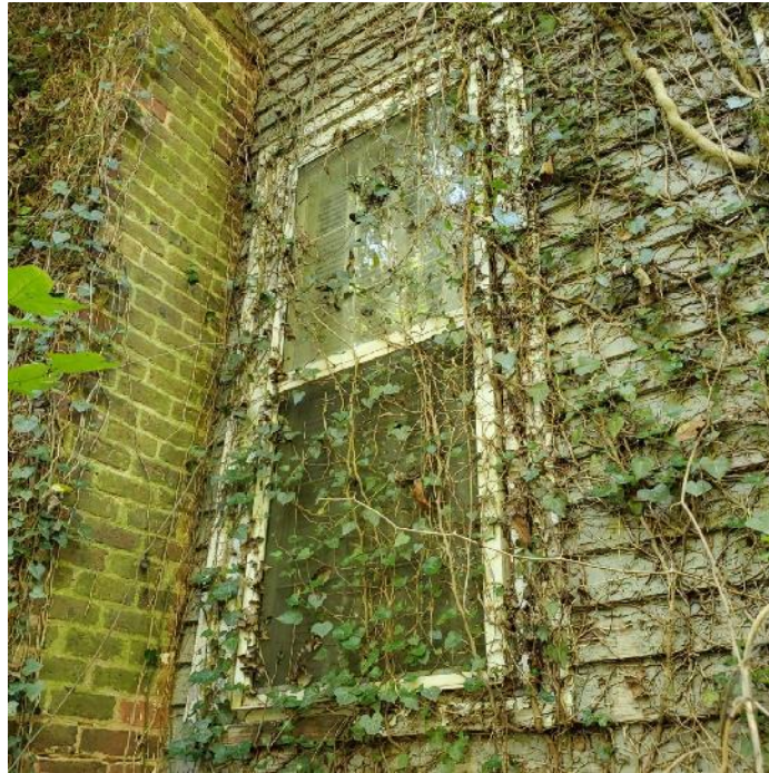
Photograph 27: Representative view of secondary hung window covers installed outboard of the original single-pane windows.
