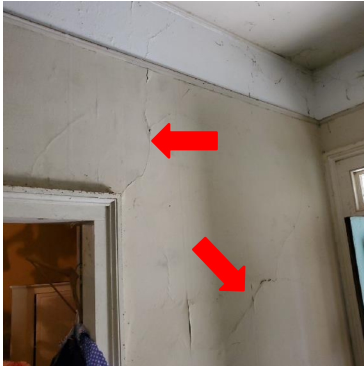
Photograph 39: Representative view of cracking within interior finishes of the original portion of the residence (arrows).
