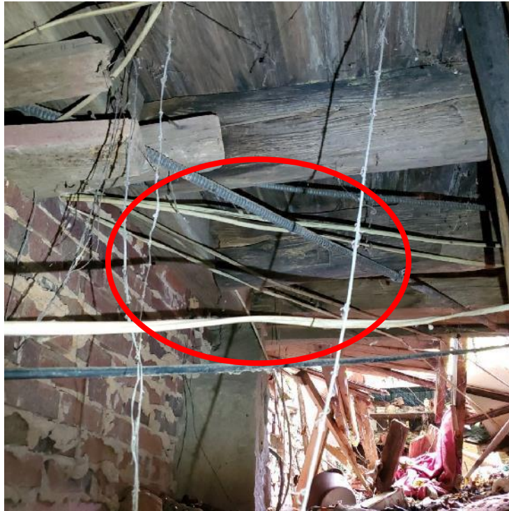
Photograph 59: View of split at notched beam end connection (oval).
