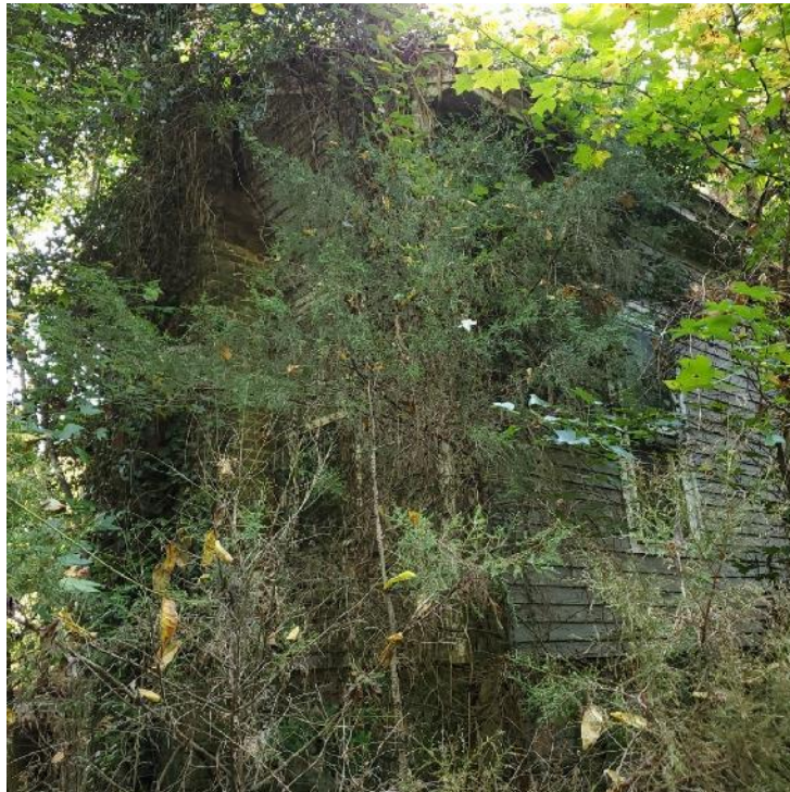
Photograph 12: View of heavy vegetative growth at rear portion of residence.
