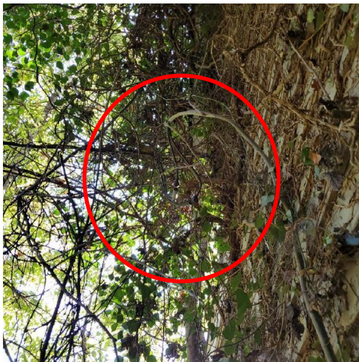
Photograph 14: View of vegetative growth at city electric line to residence (oval).
