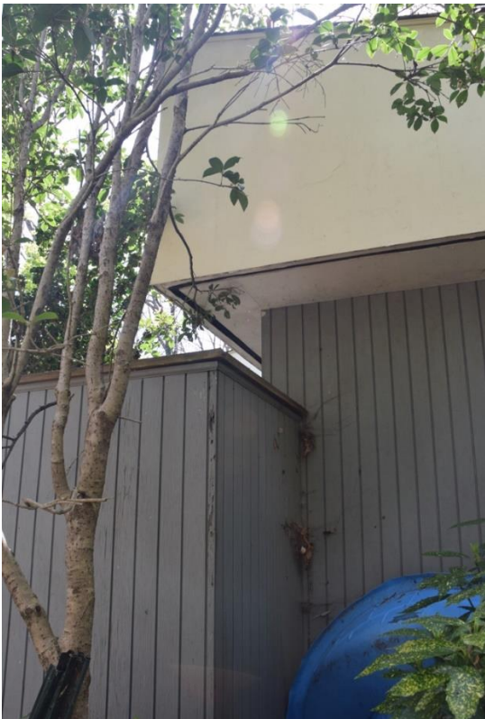
A wall sheathed in T1-11 extends from the east elevation to the carport, enclosing the courtyard. The wall rests on a brick foundation and is topped with a copper cap.
