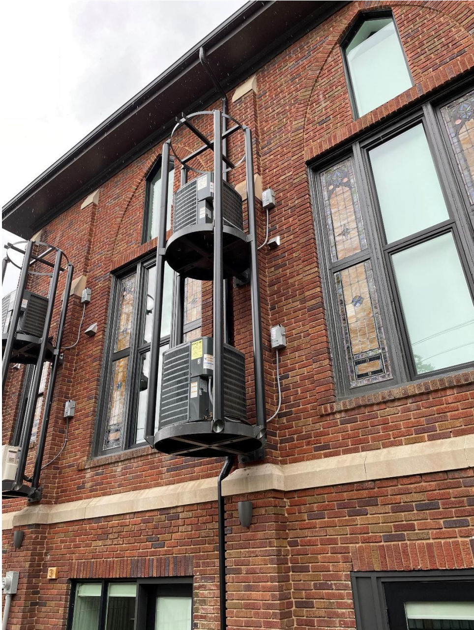
Figure 13 Typical heat pump surround at east elevation. The metal sheathing had not been applied at the time of this report's completion.
