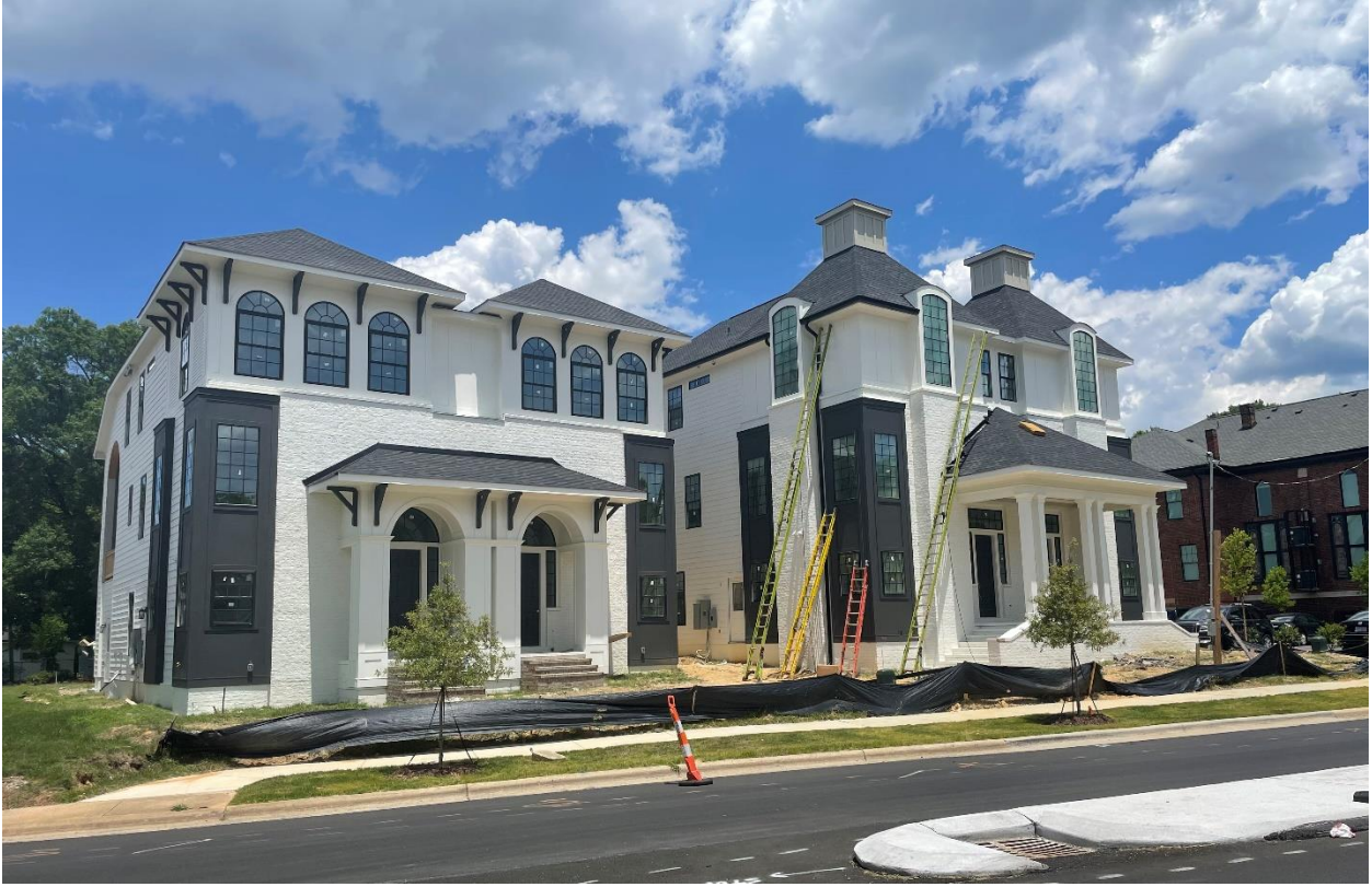
Figure 6 The duet units under construction. They are located on the western portion of the property along Parkwood Avenue.
