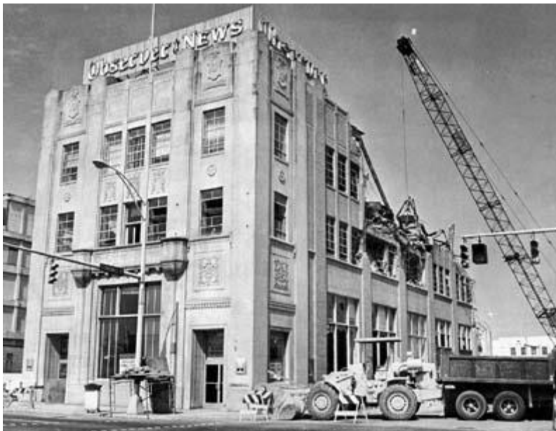
The Art Deco style Charlotte Observer/Charlotte News Building was demolished in 1970 with no serious attention having been given to its preservation. Preservation has never been a vital part of comprehensive planning in Charlotte.
