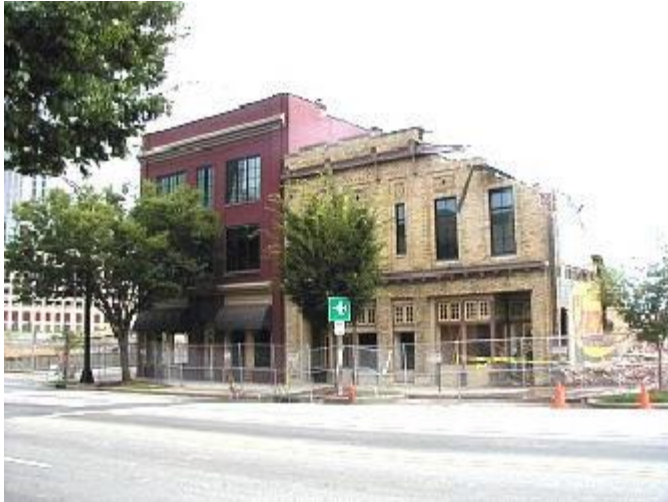
This July 2003 photograph shows two historic buildings being demolished on E. Trade St. to make way for the new Uptown arena. Efforts to save the building were "too little, too late."
