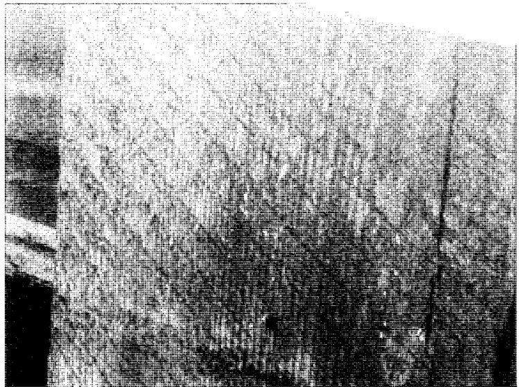
Saw marks on vertical timber of Wing (just above front porch roof).
