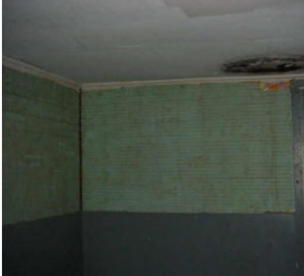
The schoolhouse's interior reveals a lowered ceiling and beaded-board behind the wall boards.
