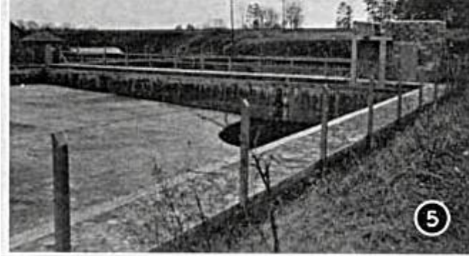
Filtration System for the "Negro Public Swimming Pool."
